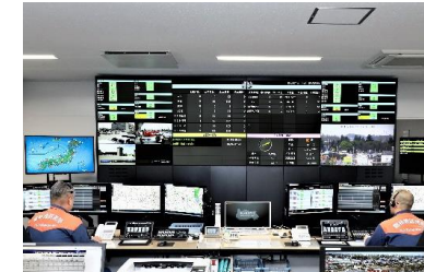
Fire and emergency communication command system
