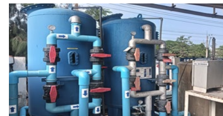
Oil skimmer and carbon filter tank used in wastewater processing systems (TCFG)
