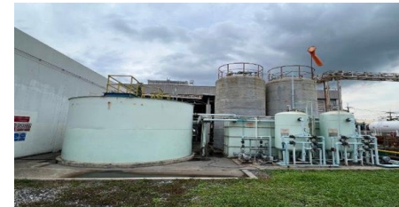
Chemical wastewater processing facilities (FGT)
