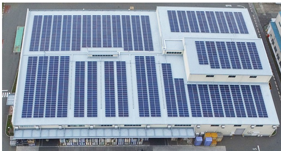
Solar panels (Operation from December 2017)
