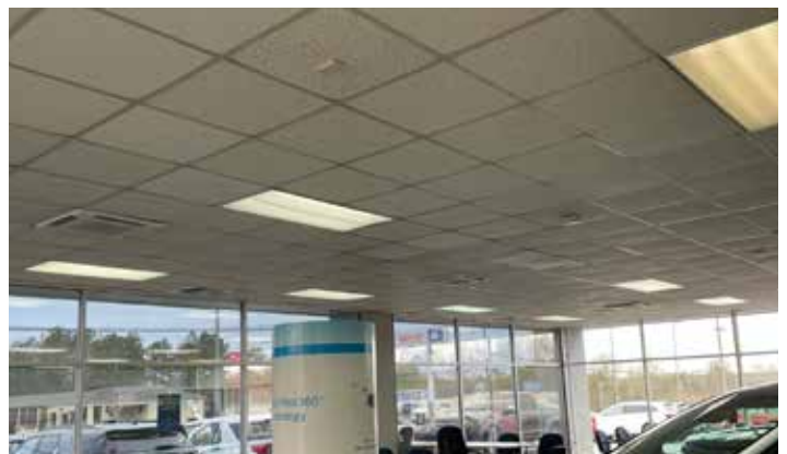
Below ↓: Six 24,000 BTU/h Grid-Fit Compact Cassettes were installed in the showroom.
