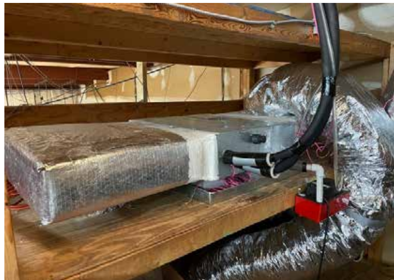
Above ↑: 24K Mid-Static Ducted Air Handler installed for the common areas of the dealership
