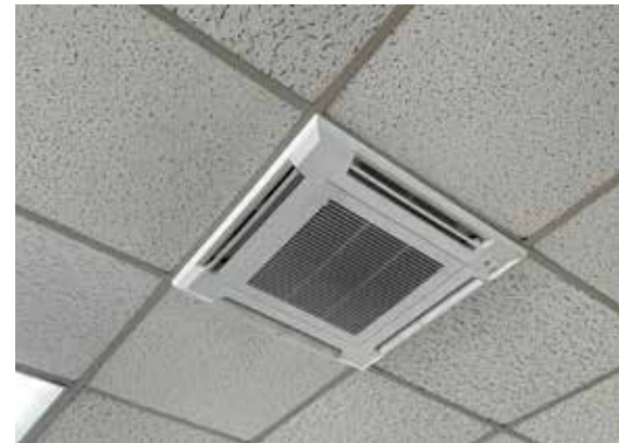
Six 24,000 BTU/h Grid-Fit Compact Cassettes were installed in the showroom.
