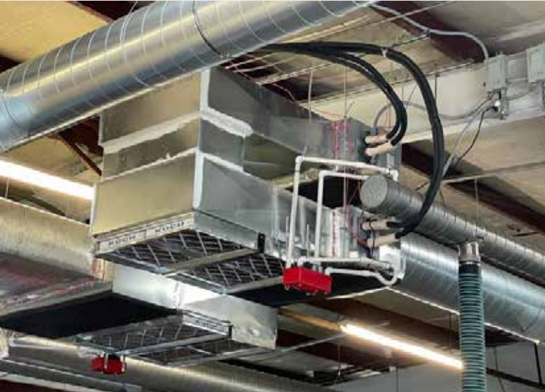
24K Mid-Static Ducted Air Handler installed for the common areas of the dealership
