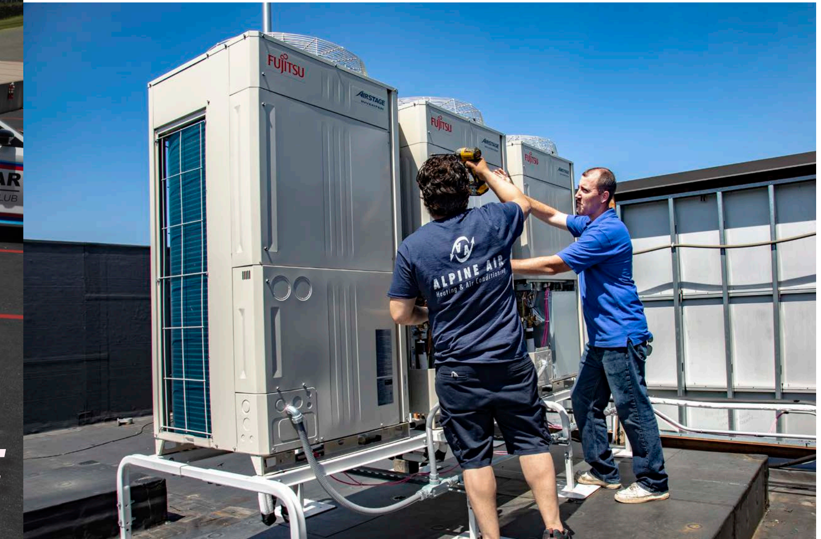
Erik Nieto and Tom Bogert check a VR condensing unit.
