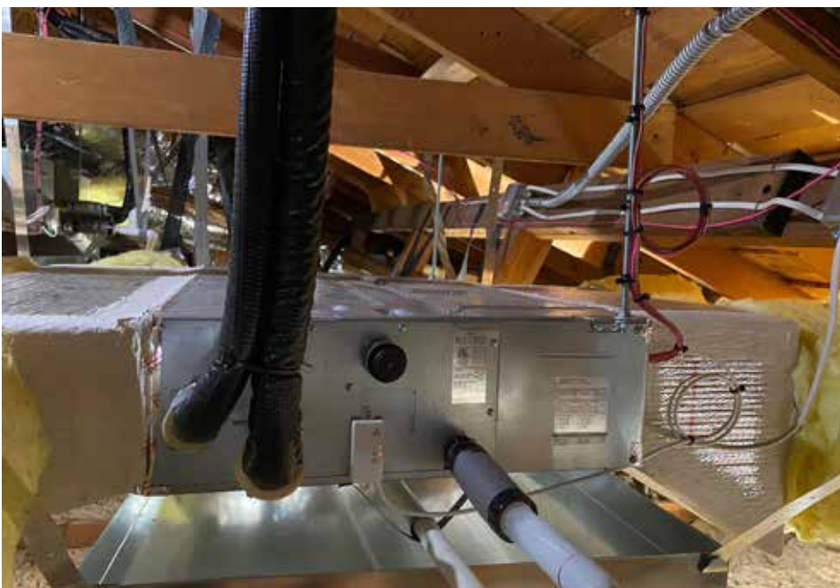
Compact Slim Duct Indoor unit with optional wi-fi module is installed.
