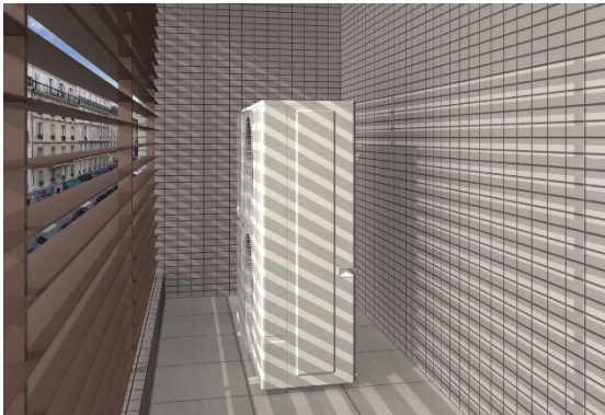
AIRSTAGE J-III L series model installed on a balcony covered by an external louver (Image)
